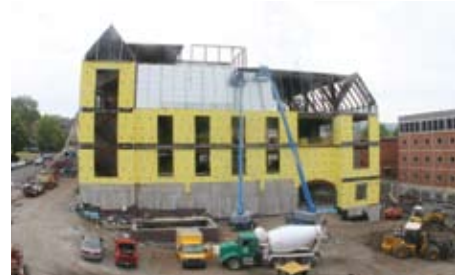
Exterior insulation was applied to the building in the spring and summer of 2007.
